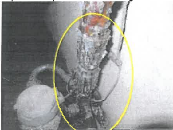
leaking on main
