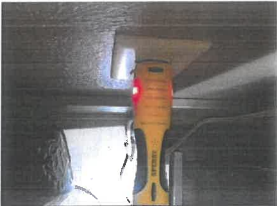
3-prong ungrounded outlets.
