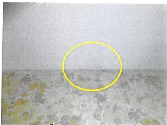
moisture related stains
