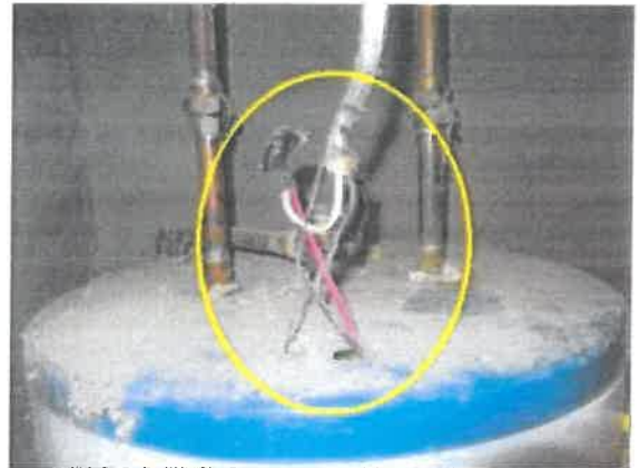
wiring should be in the water heater housing
