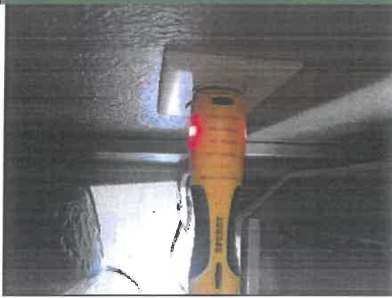
3-prong ungrounded outlets.
