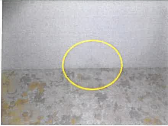
moisture related stains
