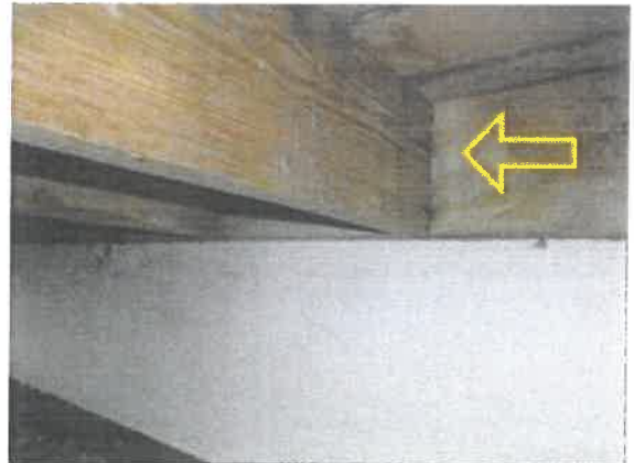
missing joist hangers
