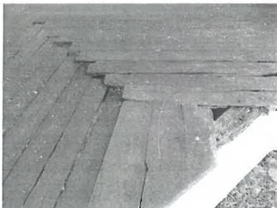
Deteriorated floor boards
