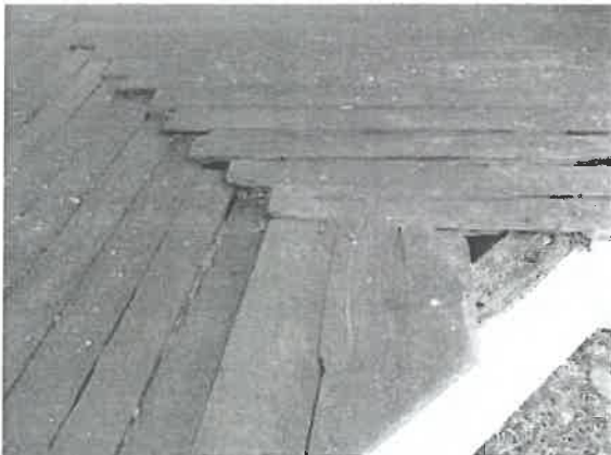
Deteriorated floor boards
