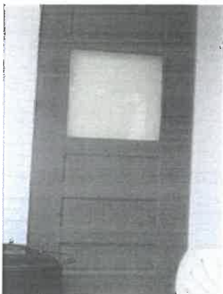
porch door sealed, not in use
