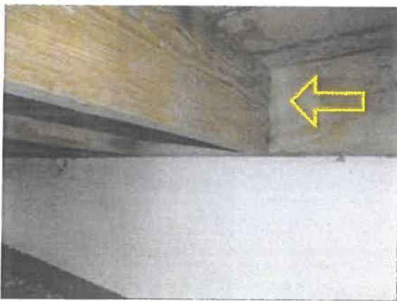
missing joist hangers
